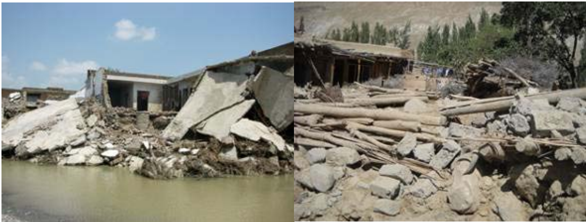
Image 3 & 4 (left to right): These images depict the level of infrastructural damage incurred by the floods in Kharko Ganche.
